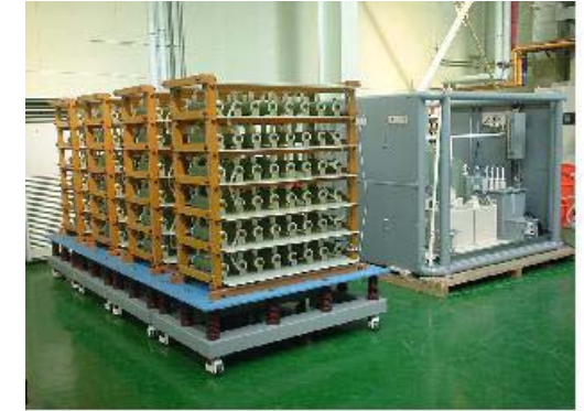
Capacitor Filter Deck & Crowbar Resistor Load
